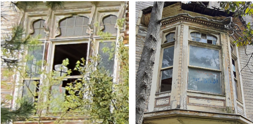
Fig. 13. Rectangular arched windows at a 1:2 proportion and underlying rectangular decorative cartouche work in the Orientalist-Moorish style, that is profusely used throughout the kiosk (Author)
