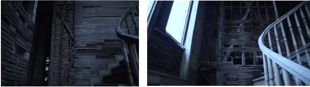
Fig. 15. Right: Bağdadi slats on the wooden frame system. Left: Brick-filled wooded frame system with bağdadi (İbrahim Akgün)
