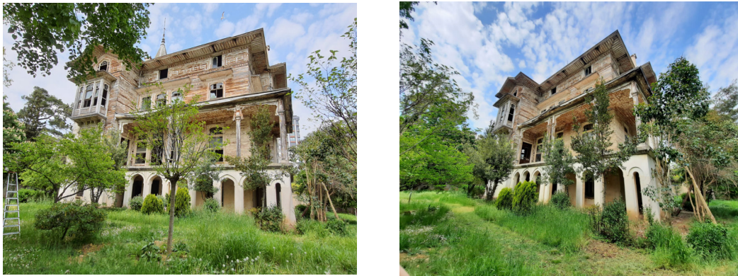
Fig. 9. Above and below: The wooden-posted veranda overlooking the sea on the ground floor (Author)
