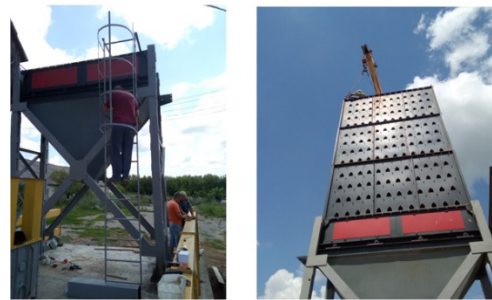
Fig. 7. Installation of the column type grain dryer with the capacity of 5 t/h
