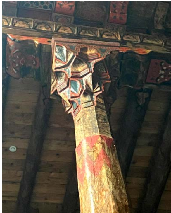
Fig. 17. Above: Wooden columns with muqarnas capitals and the wooden ceiling (Mustafa Cambaz) . Below: Wooden columns with muqarnas capitals (Author)
