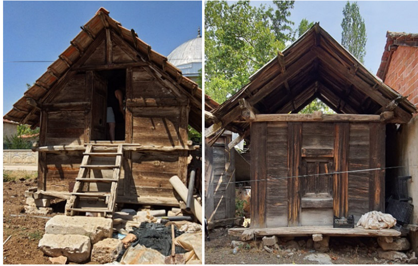
Fig 5. Granaries consisting of a single space, with and without stairs in front (Author)
