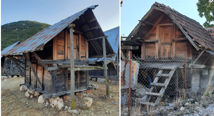
Fig. 19. Supporting wooden buttresses of the steep gabled roof. Granaries in the villages of Kaş Bezirgan and Elmalı Plains (Author)
