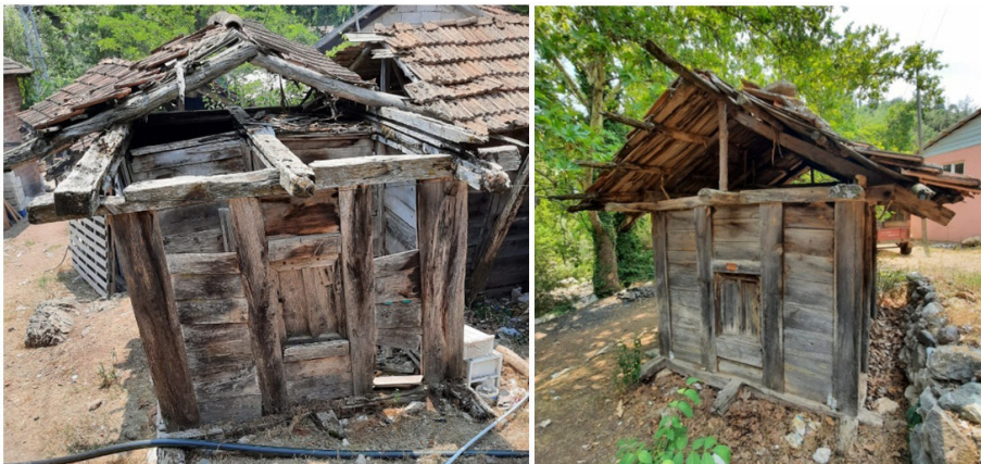
Fig 20. In the construction of the roof walls, the ends of the frame girders of the head beam and of the tie beams are projected outwards at the corners and forward in the middle, all elements of the roof being joined together using the “kurt boğazı” joint system (Author)
