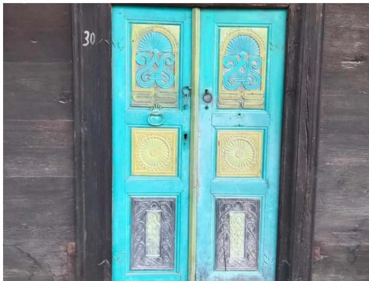
Fig. 14. Example of decorative entrance doors. Samsun Kavak Bekdemir Village Mosque (Source: Kavak District Governorship)
