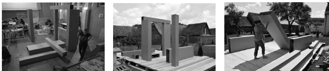
Fig. 11. Work in progress on the prototype: execution and assembling of the modules in the workspace and placing them in their final position in the courtyard of the household (Photo: Thomas Gronegger, 2016)
