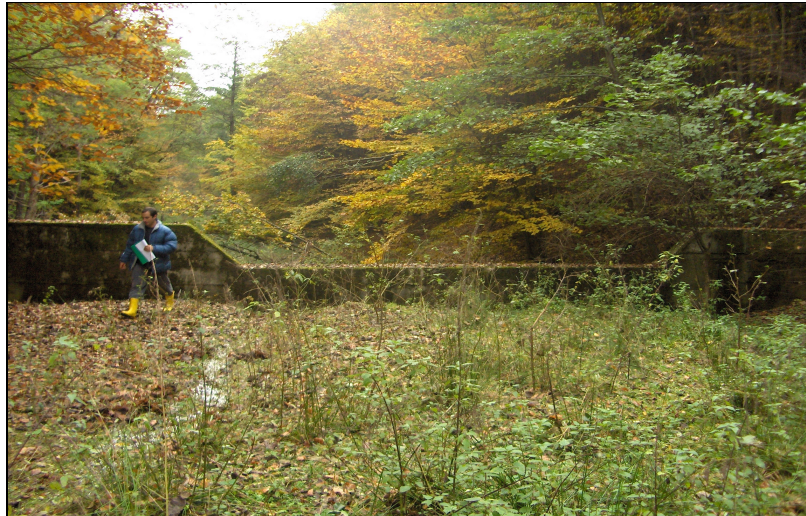
Fig. 1. The consolidation of a torrential riverbed through the mean of hydrotechnical works, in the Upper Cărcinov watershed. Photo: Tudose, 2009
