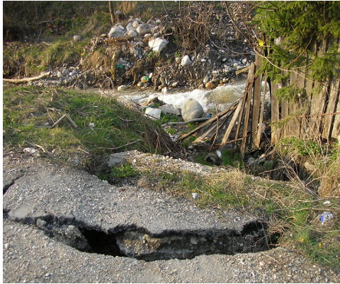
Fig. 1. Road degradation DC 51
