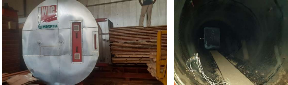
Fig. 1. Thermal vacuum system and interior view of the thermos-vacuum plant
