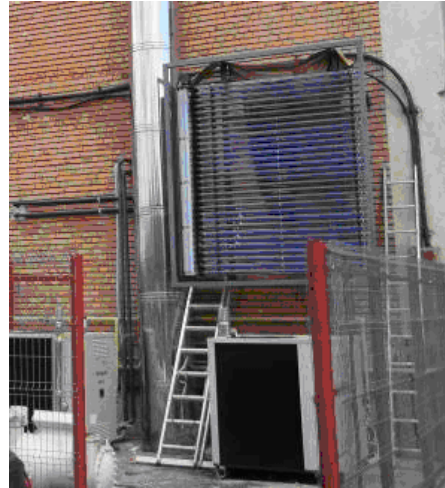
Fig. 9. The heat pump and the chiller platform
