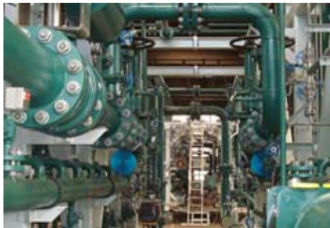
Fig. 1. Pipes with compensators
