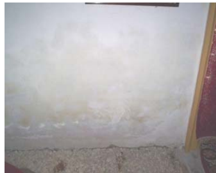
Fig. 1. Blooms and coloured spots on the plaster
