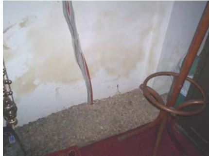
Fig. 2. Coloured spots on the coating, caused by migration of salt from walls
