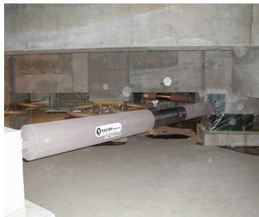
Fig. 11. Installed viscous damper [1]
