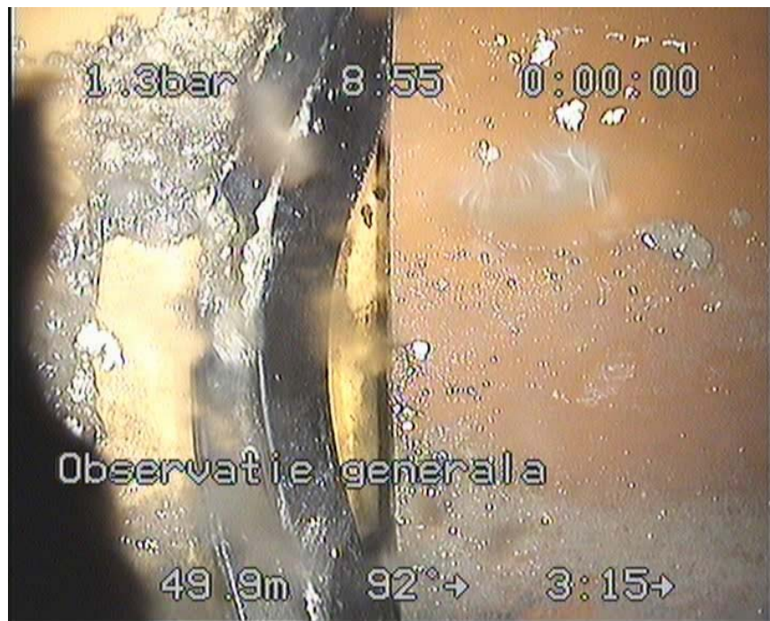
Fig. 3. Rubber gasket expelled from groove in a PVC pipe joint
