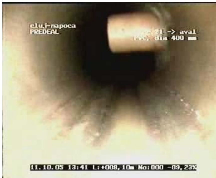
Fig. 4. Protruding lateral inside sewer main prevents the camera robot to advance along the pipe [2]
