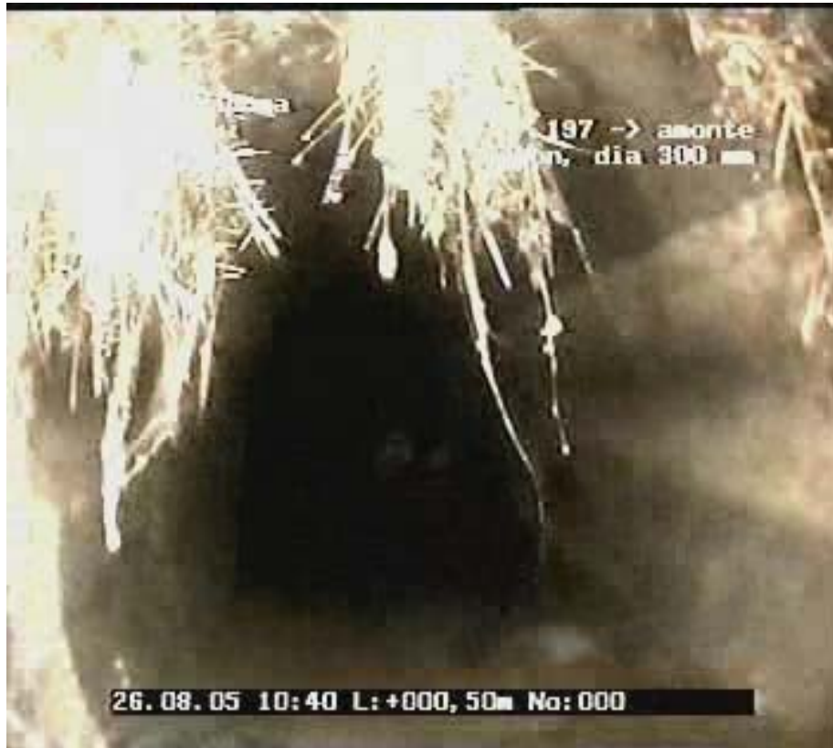
Fig. 5. Early stage of roots penetrating inside concrete sewer pipe [2]
