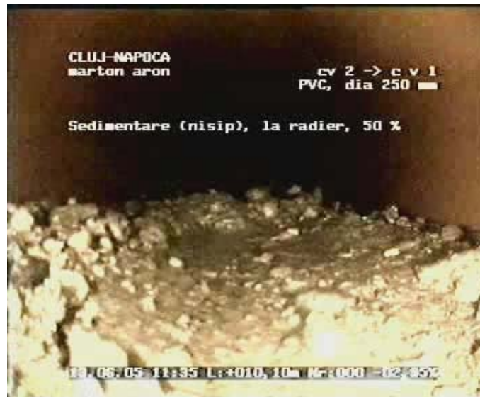
Fig. 6. Deposits of sediments – 50% of the pipe cross sections is unusable due to sediments
