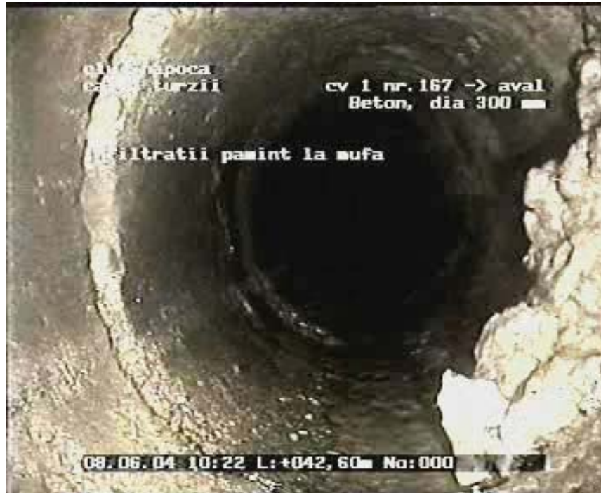
Fig. 2. Faulty joint in a concrete sewer section allowing soil to enter inside the pipe (in the right side of the image)
