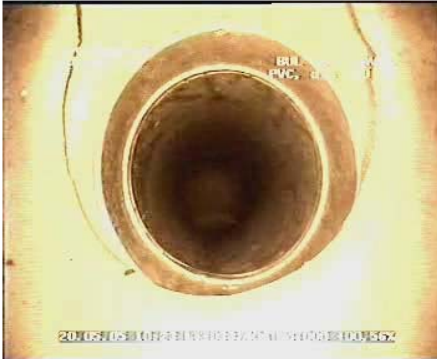
Fig. 1. Cracks in the wall of a PVC sewer main at a lateral joint due to uneven soil compaction and the lateral acting as a lever
