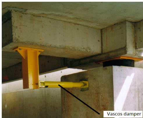
Fig. 2. Viscous damper installed in base isolated structure
