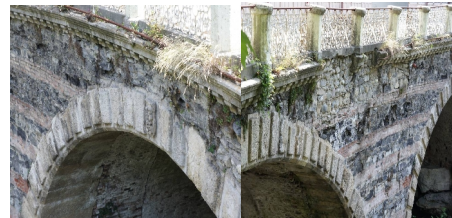
Fig. 9. Vegetation, damaged masonry elements
