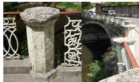
Fig.10. Ornaments are missing
