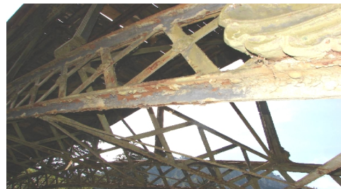
Fig. 6. The corroded arches
