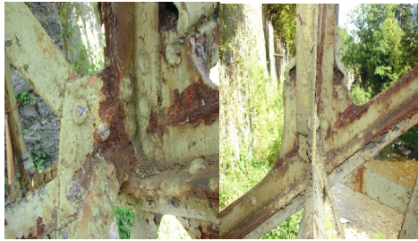
Fig. 7. Corroded joint and vertical member
