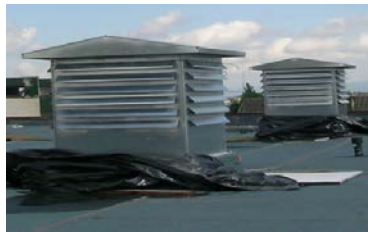
Fig. 5. Turrets mounted on roof for exhaust air
