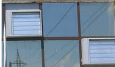
Fig. 4. Two of grilles fitted in front for introducing air
