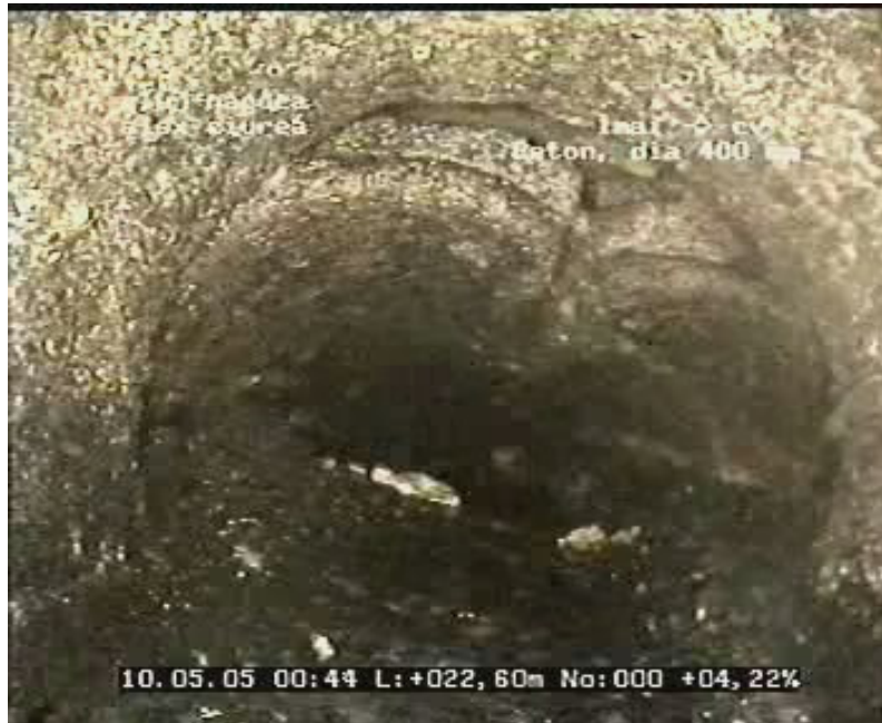
Fig. 1. Total collapse of a concrete sewer pipe. The sewer section is impossible to use. The picture illustrates the faults included in the first category.
