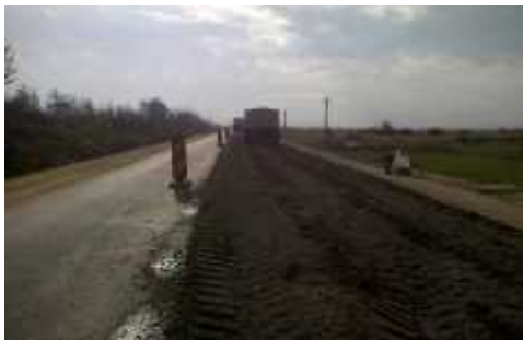
Fig. 7. Spreading the hydraulic road binder Doroport TB25 in the lab recipe percentage
