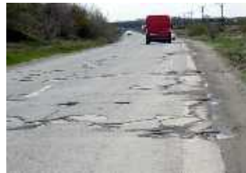
Fig. 1. Degraded layers on DN 66 between Targu Jiu - Bumbesti Jiu
