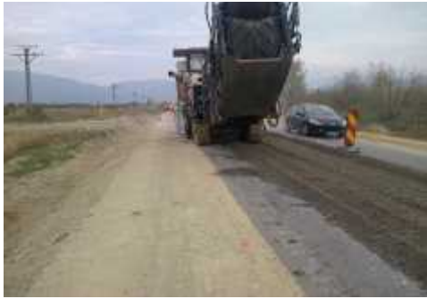
Fig. 6. Milling the existing layers and placing them for the stabilization in a belt
