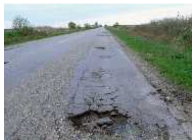
Fig. 2. Degraded layers on DN 66 between Rovinari and Targu Jiu
