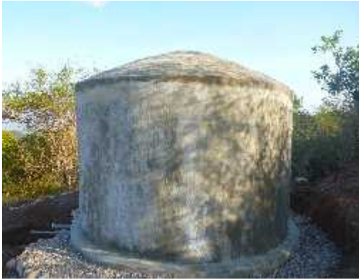
Fig. 6. Water reservoirs with ferrocement
