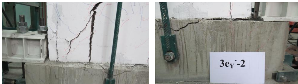
Fig. 6. Level of damage encountered in beam foundation and at the base of the wall
