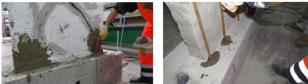
Fig. 4. Phases from strengthening procedure - inserting steel rods and repairing the damaged concrete with high performance repairing grouts
